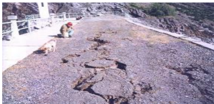
Figure 12: Tension cracks on Cogoti Dam crest associated earthquake in 1997
