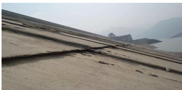
Figure 8: Damages of concrete slab Zipingpu dam after Wenchuan earthquake in China
