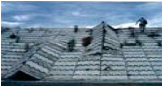
Figure 9: Buckling of canal lining elements In the 21 September 1999 Chi-Chi earthquake in Taiwan
