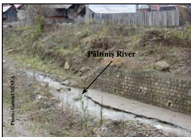
Photo 1 Hydrotechnical work destroyed by the flood from July 20 th 2002 (near the confluence of the Păltiniș with the Bâsca River)
