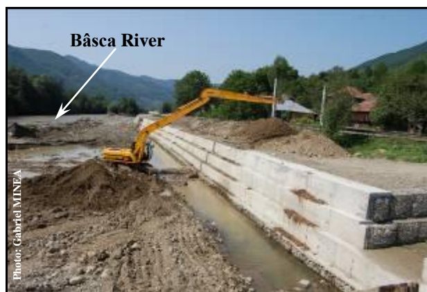
Photo 2 New hydrotechnical arrangements (gabion baskets) on the Bâsca River (august 10 th 2010)
