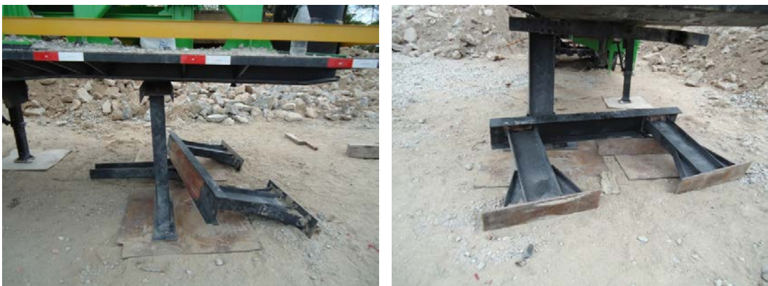
Fig. 6. (a) improvised support for the truck; (b) the metal piece that fell on the employee.
