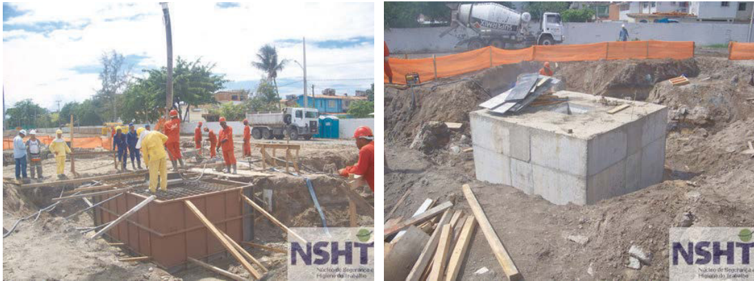
Fig. 3. (a) concrete blocks for crowning the piles; (b) concreted crowning block to connect the stakes to the pillar.
