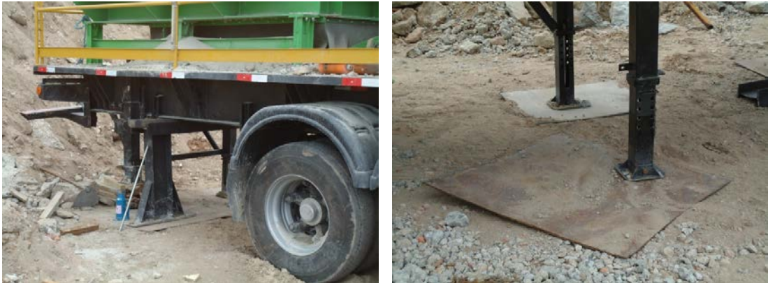
Fig. 5. metal parts for fixing the mobile equipment.
