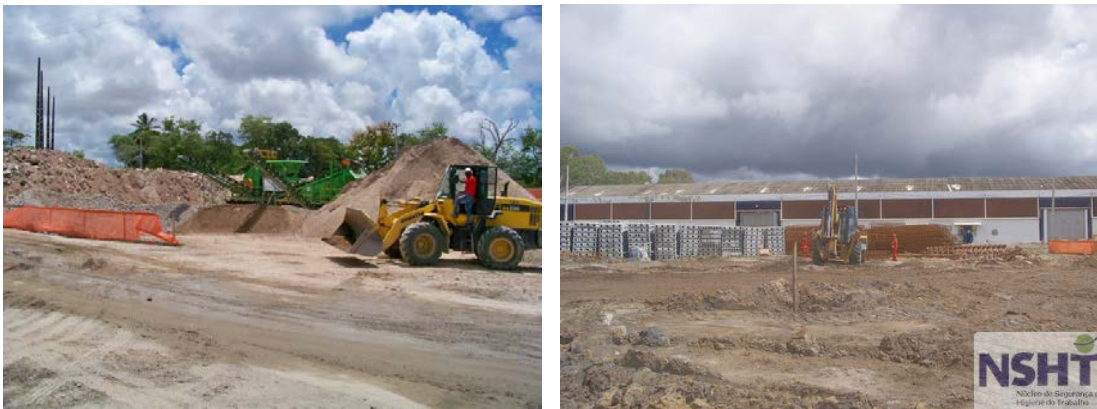
Fig. 1. (a) area for the recycling of solid waste; (b) sheds of the old factory before demolition.
